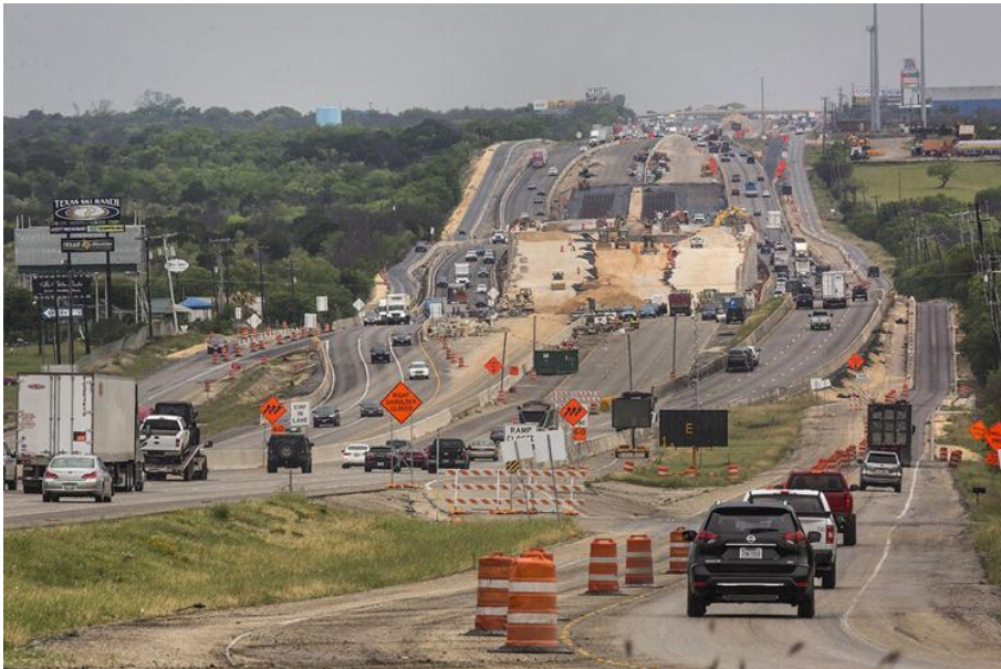
Figure 1. Construction takes place on I-35 on Tuesday, April 27, 2021. (Source: Compton, 2021, retrieved from https://herald-zeitung.com/community_alert/article_c3dc462c-a942-11eb-acf5-3b3987212749.html )
